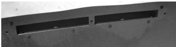
Fig 2b - Flue Restrictor Baffle Not Fitted
