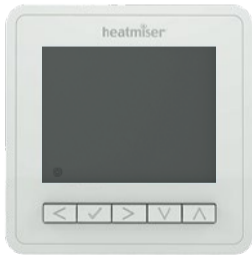
Thermostat completely OFF
